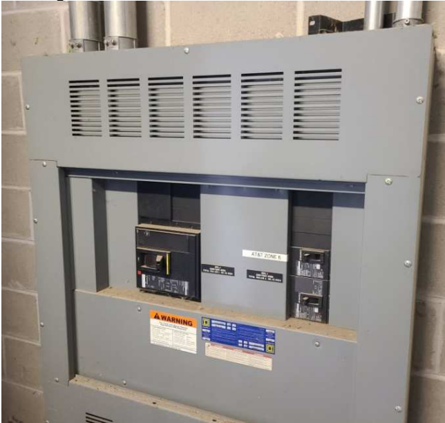
Existing Distribution Panel
